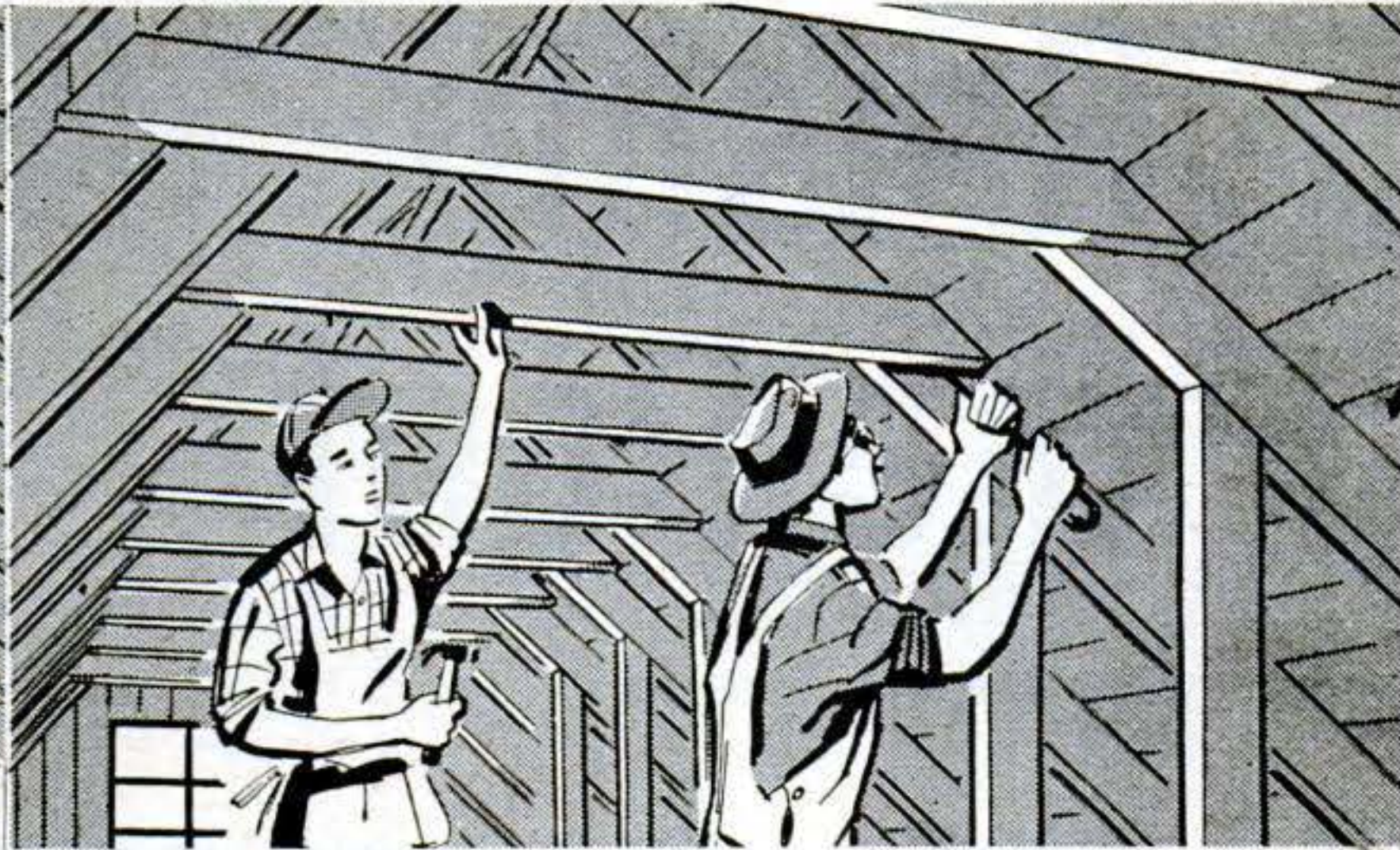
2 COLLAR BEAMS , which tie rafters together, are removed in area the dormer will occupy. Next the ridge pole is sawed from outside at each end of the dormer space.
